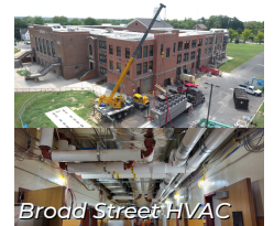
Broad Street HVAC
